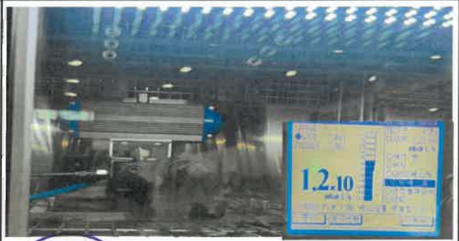
Leakage Stem Seal: 1.2 E-06
