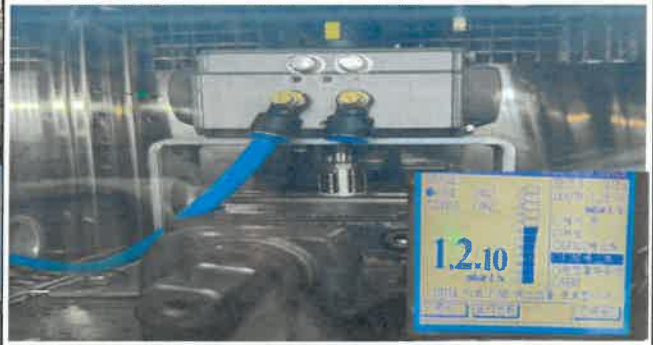
Leakage Stem Seal: 1.2 E-06
